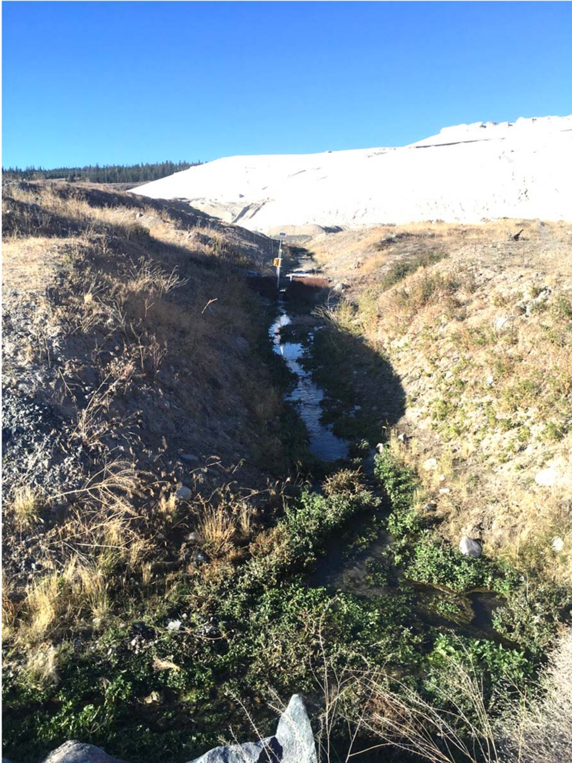
Photo II-A-24 UVD/LVD Drain Measuring Weir (LL—FS-02) (LL-2017-22)
