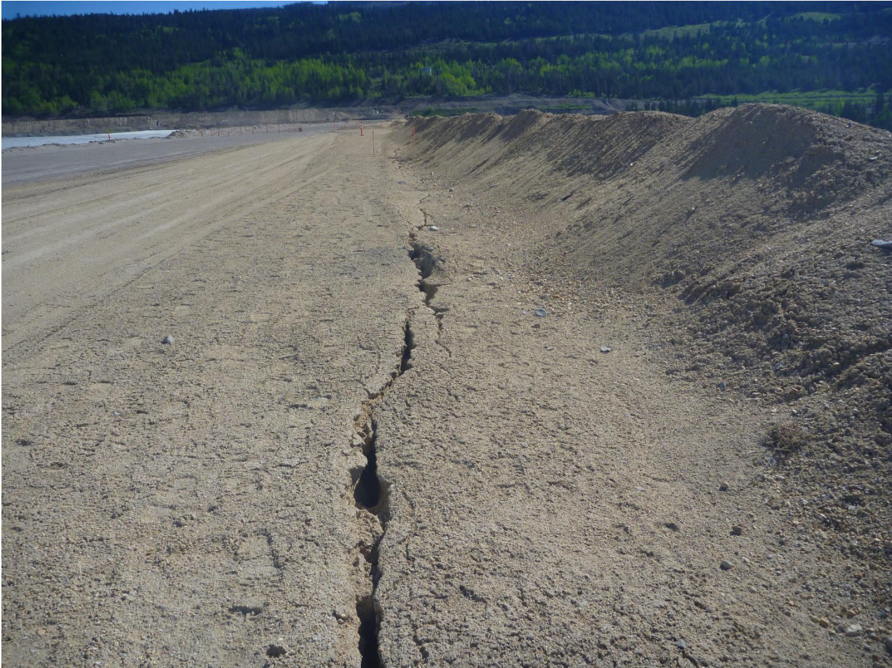
Photo 4 – Cracking on the u/s edge of SG2 zone at approx. Sta. 1+550
