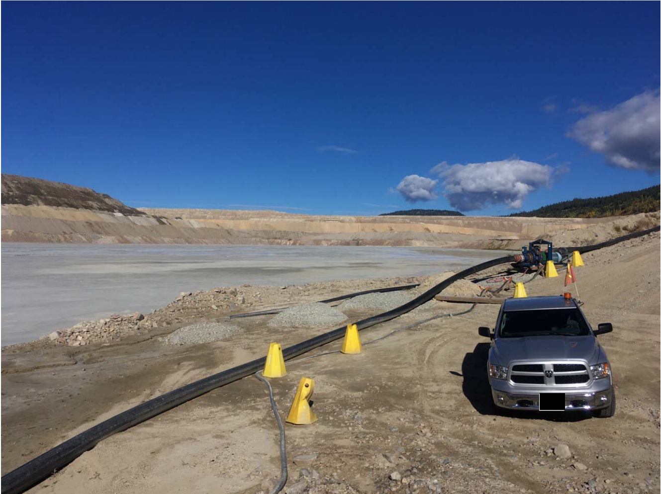
Photo II-D-3 Outflow pump location, facing H-H Dam (northwest) (ML-2017-02)
