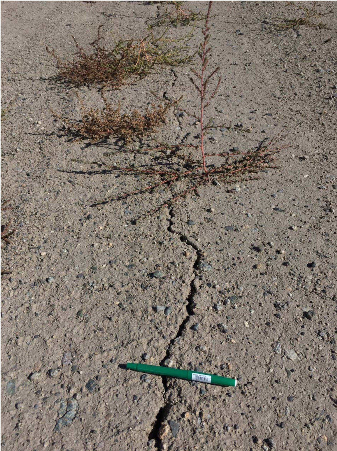
Photo II-B-5 Longitudinal cracking in Till Core Zone from Sta. 1+200 to Sta. 1+400 (not continuous) along centerline of Dam, up to 20 cm deep (HH-2017-04)
