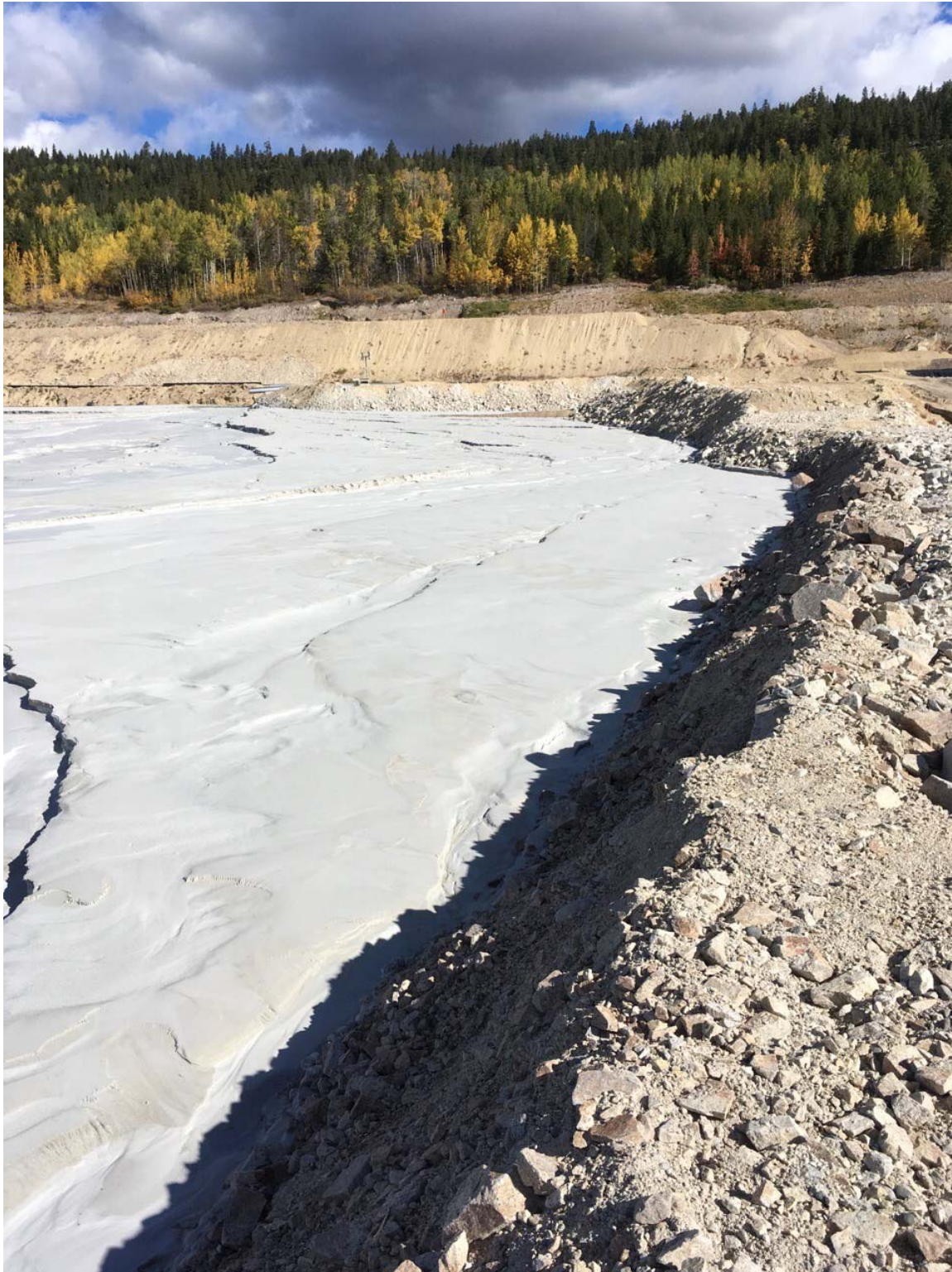
Photo II-B-8 Upstream Face of Dam - Facing Northeast; RF2/RF1 buffer zone on the upstream edge of dam crest, approx. 1 m high; available buffer is approx. 0.5 m (HH-2017-08)
