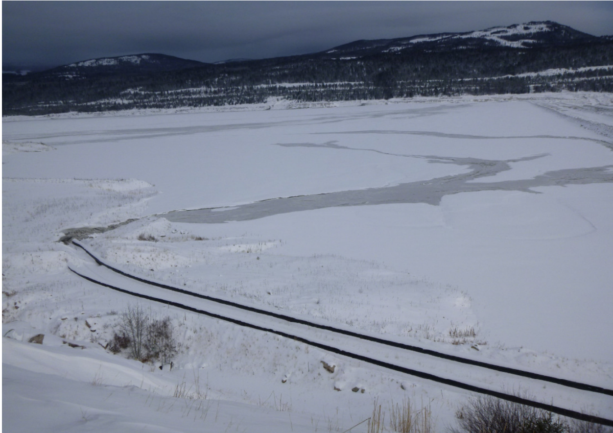
Photo 2 - Evidence of recent discharge from SS1/SS2 along/near the u/s RF2 face approximately between Sta. 0+600 to 0+750 (looking northeast).
