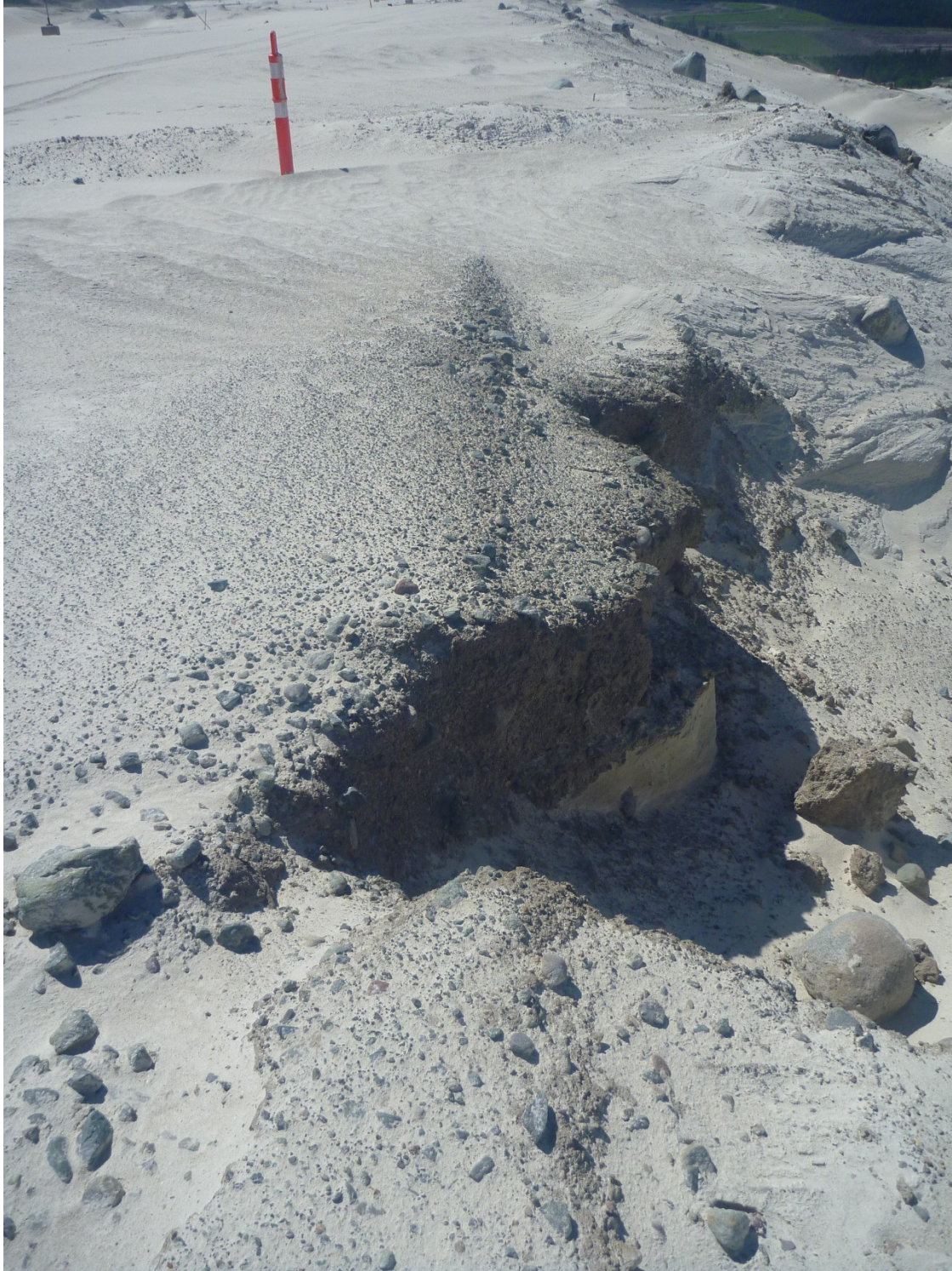
Photo 3 – Erosion feature in downstream edge of Till Core Zone at ~ Sta. 2+750
