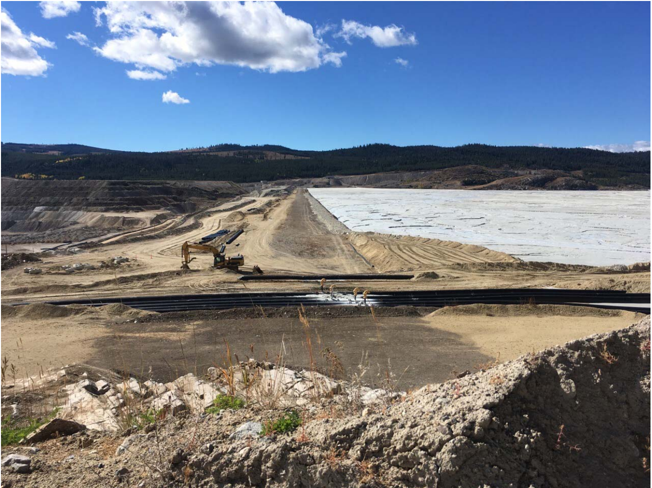
Photo II-B-2 Overview of Dam from East Abutment and Exposed Bedrock from 2015 Abutment Foundation Preparation Works (HH-2017-09)
