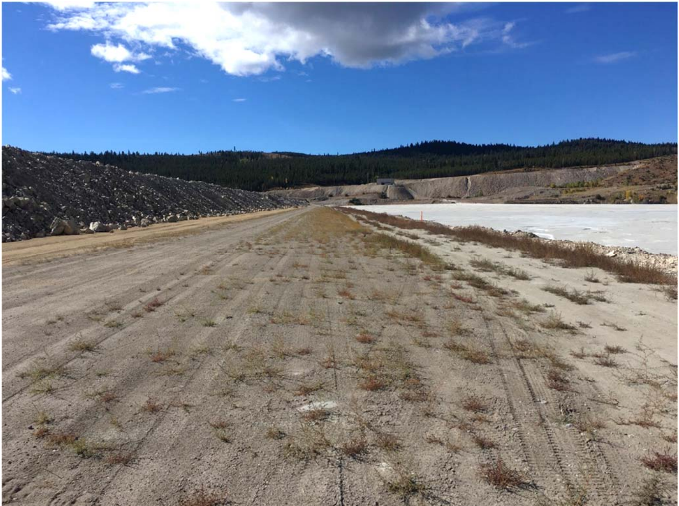
Photo II-B-3 Till Core Zone and RF1 Zone - Facing Southwest; sporadic vegetation growth (HH-2017-05)
