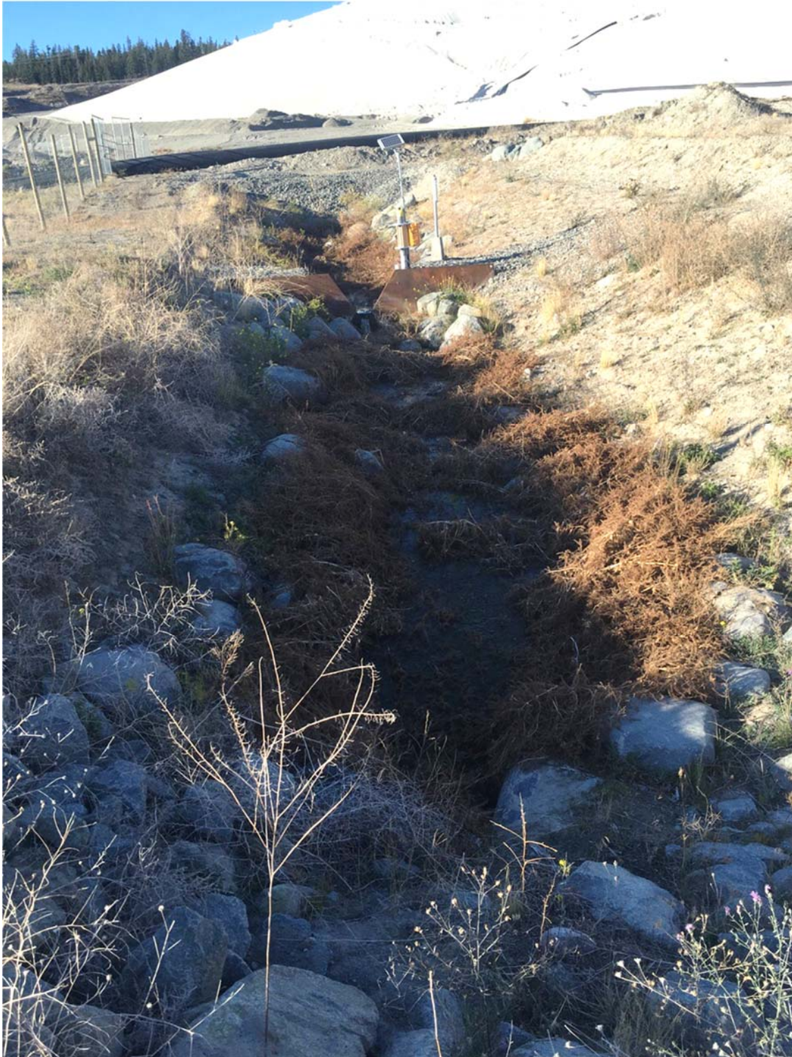
Photo II-A-23 Finger Drain No.1 Measuring Weir (LL—FS-01) (LL-2017-20)
