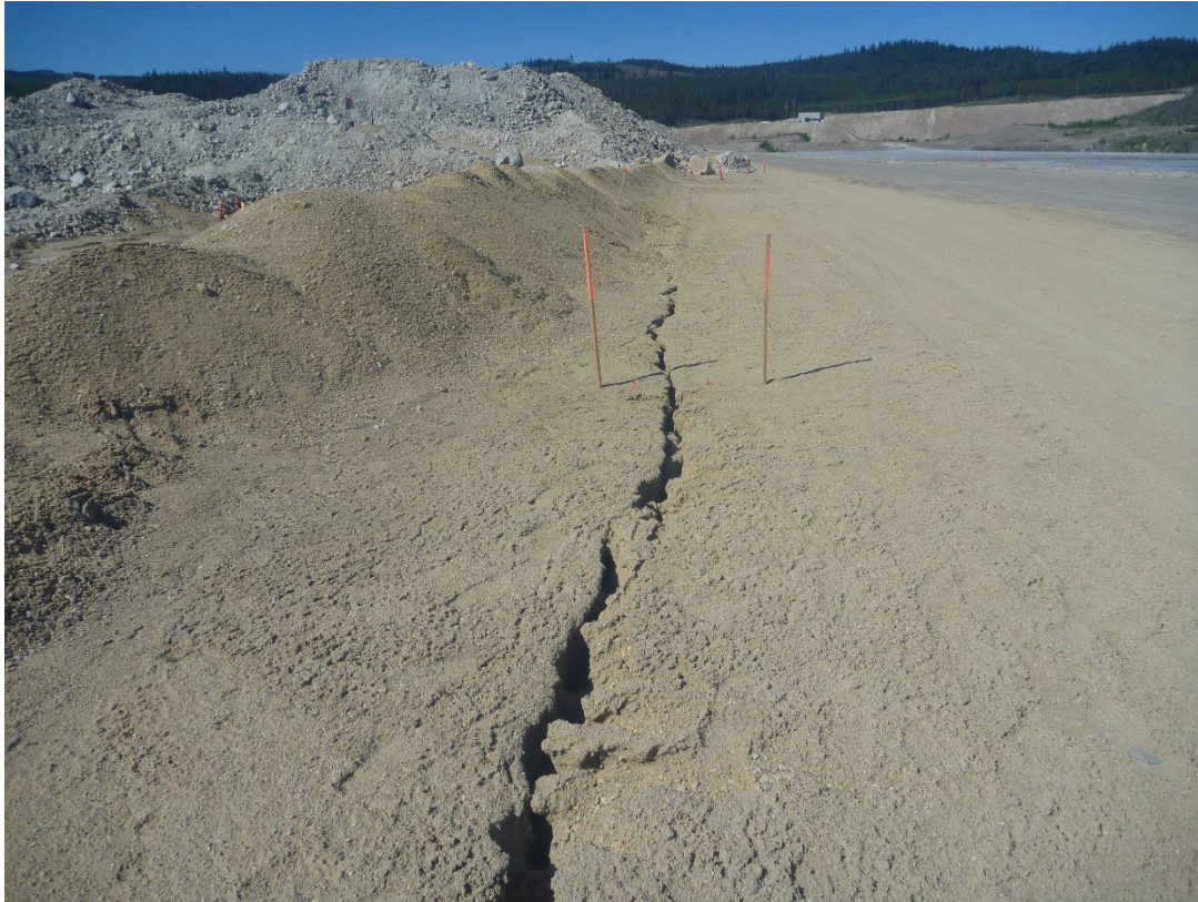
Photo 3 – Cracking on the u/s edge of SG2 zone at approx. Sta. 1+550 (facing west)
