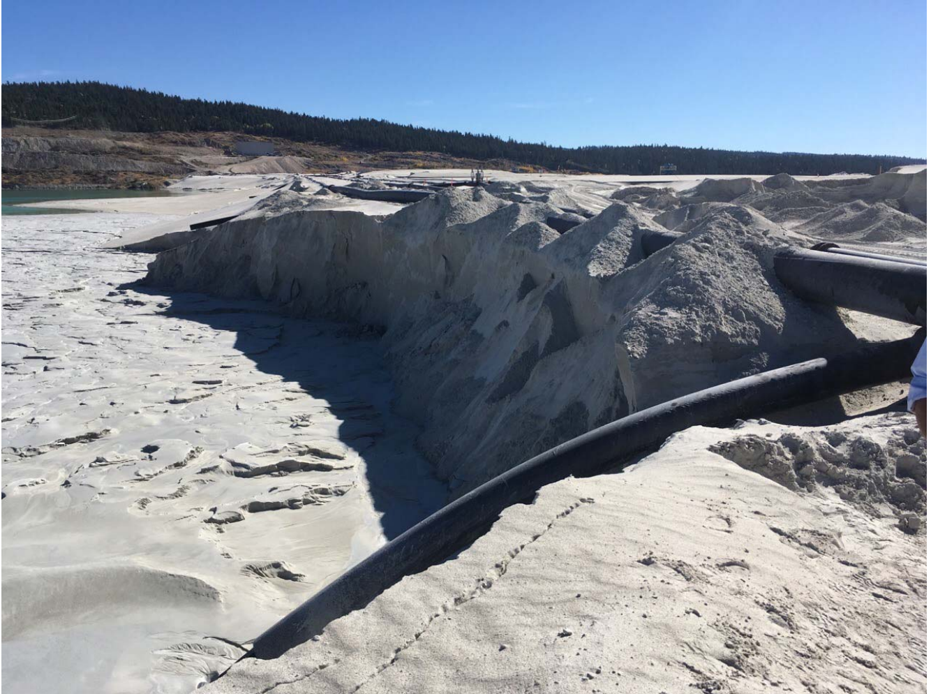
Photo II-A-6 Upstream Dam Face – Undercutting at Beaching Location – Facing North (LL-2017-10)
