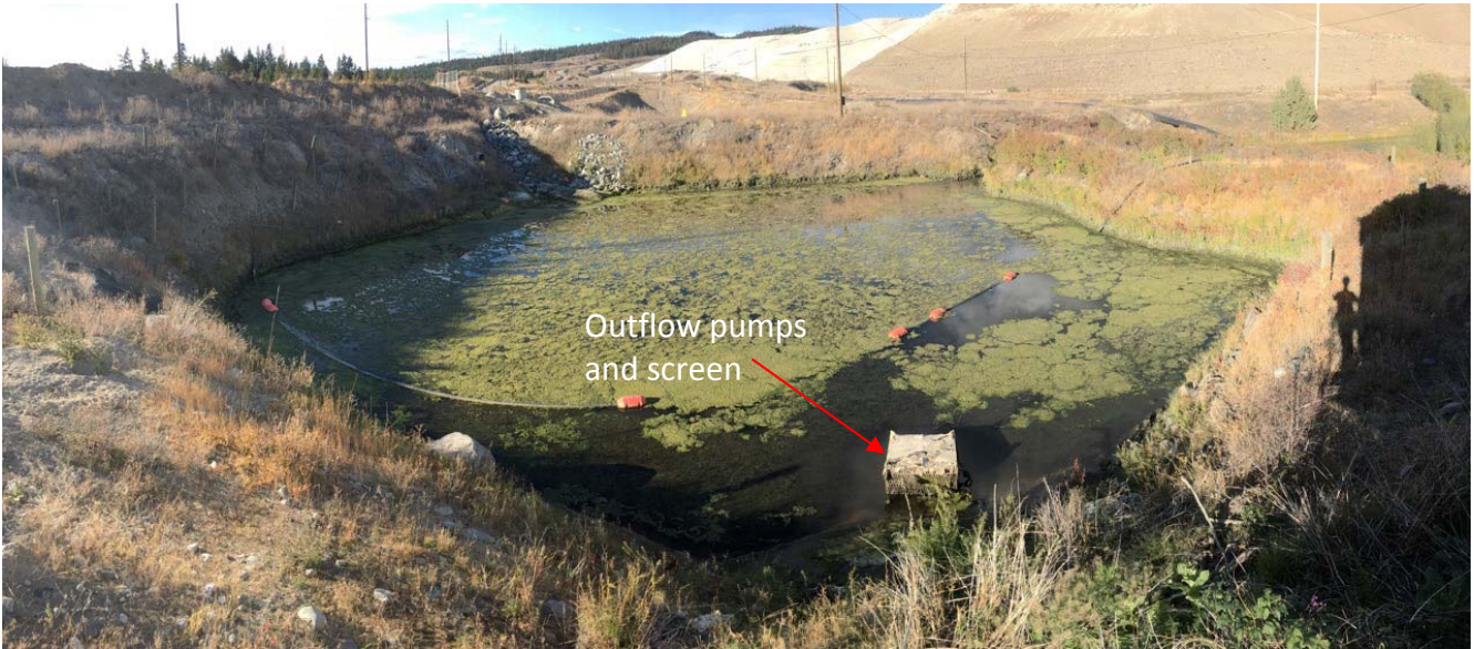
Photo II-C-13 Seepage Water Reclaim Pond – Facing North (SS-2017-09)
