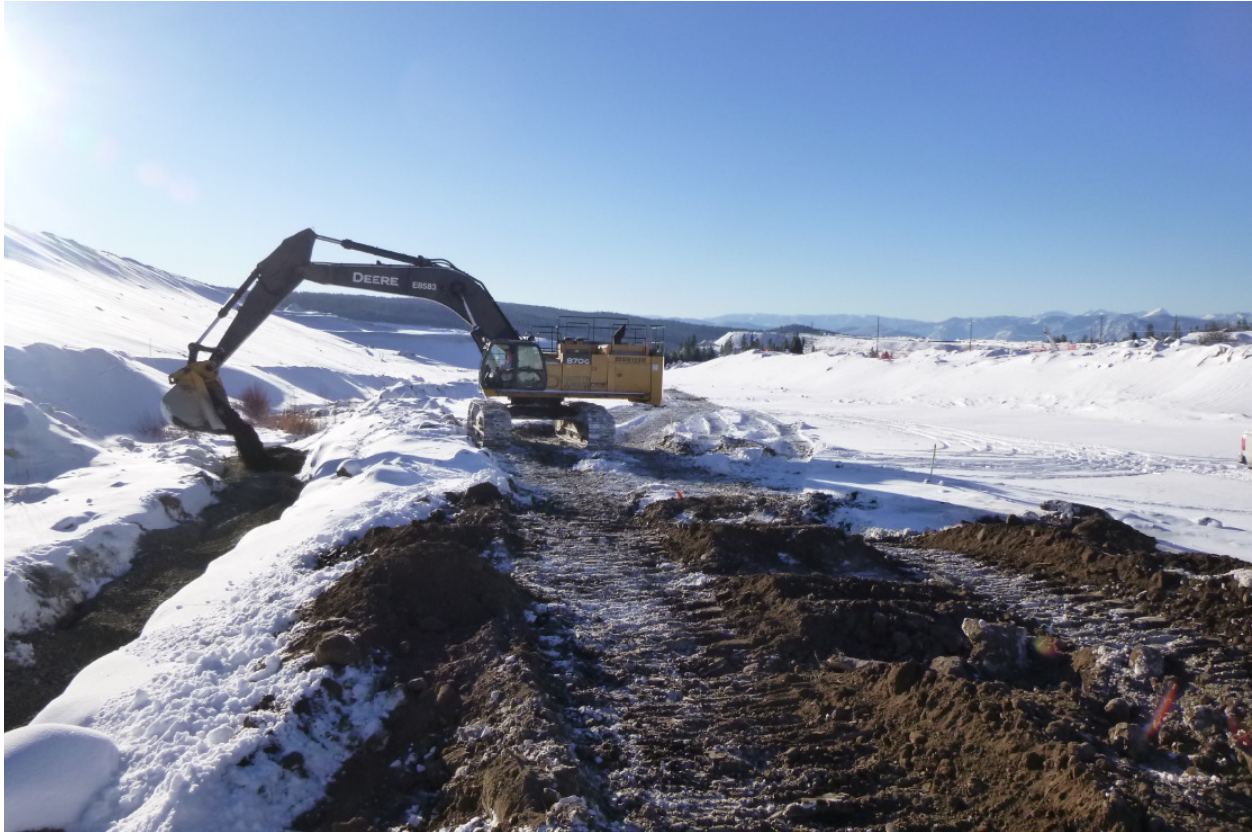
Photo 3 – Temporary ditch dug during foundation preparation works at the North Abutment (from Sta. 3+500 to ~3+570) backfilled on 17-12-20 (looking south).
