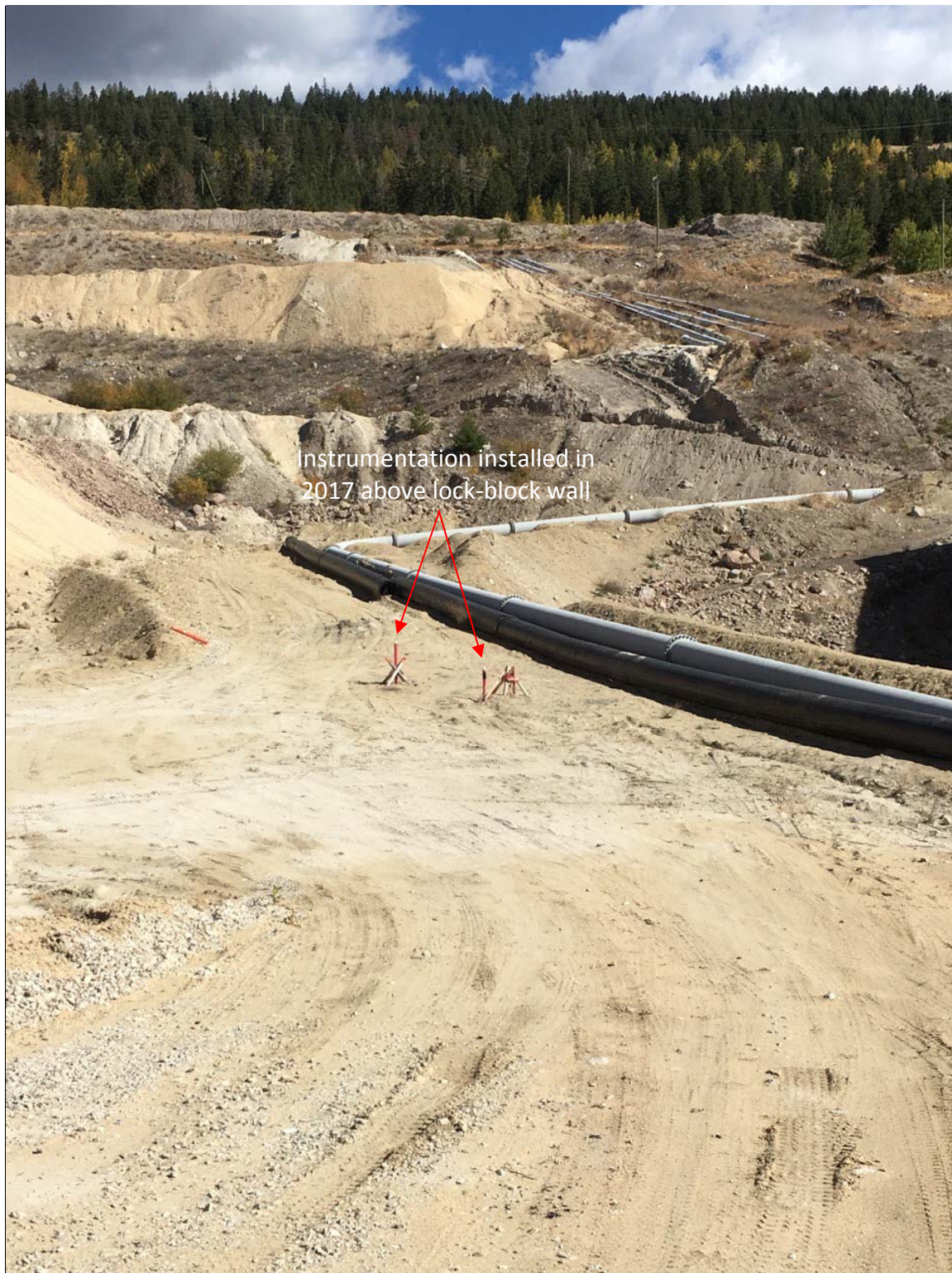
Photo II-B-13 East Abutment - Facing Northeast; new VWP, inclinometer and settlement system installed in 2017 behind the H-H Pumphouse lock-block retaining wall (HH-2017-12)
