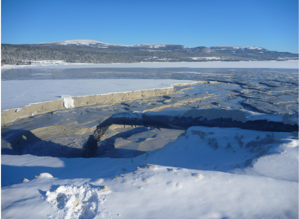
Photo 6 – Tailings discharge locations at Sta. 3+500 and 3+600 (photo taken on 17-12-20).
