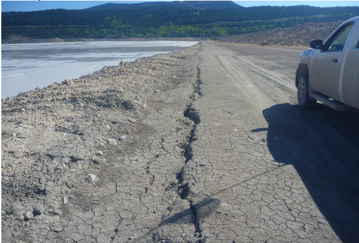
Photo 1 – Cracking at the seam between RF1 and U/S RF2 at approx. Sta. 0+800
