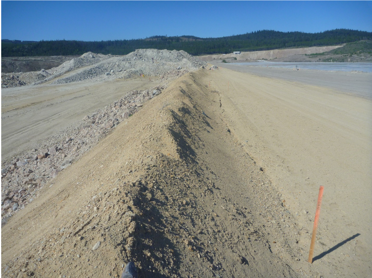
Photo 5 – Overview of cracking area on the u/s edge of SG2 zone showing height of loose safety berm (~ 4m)
