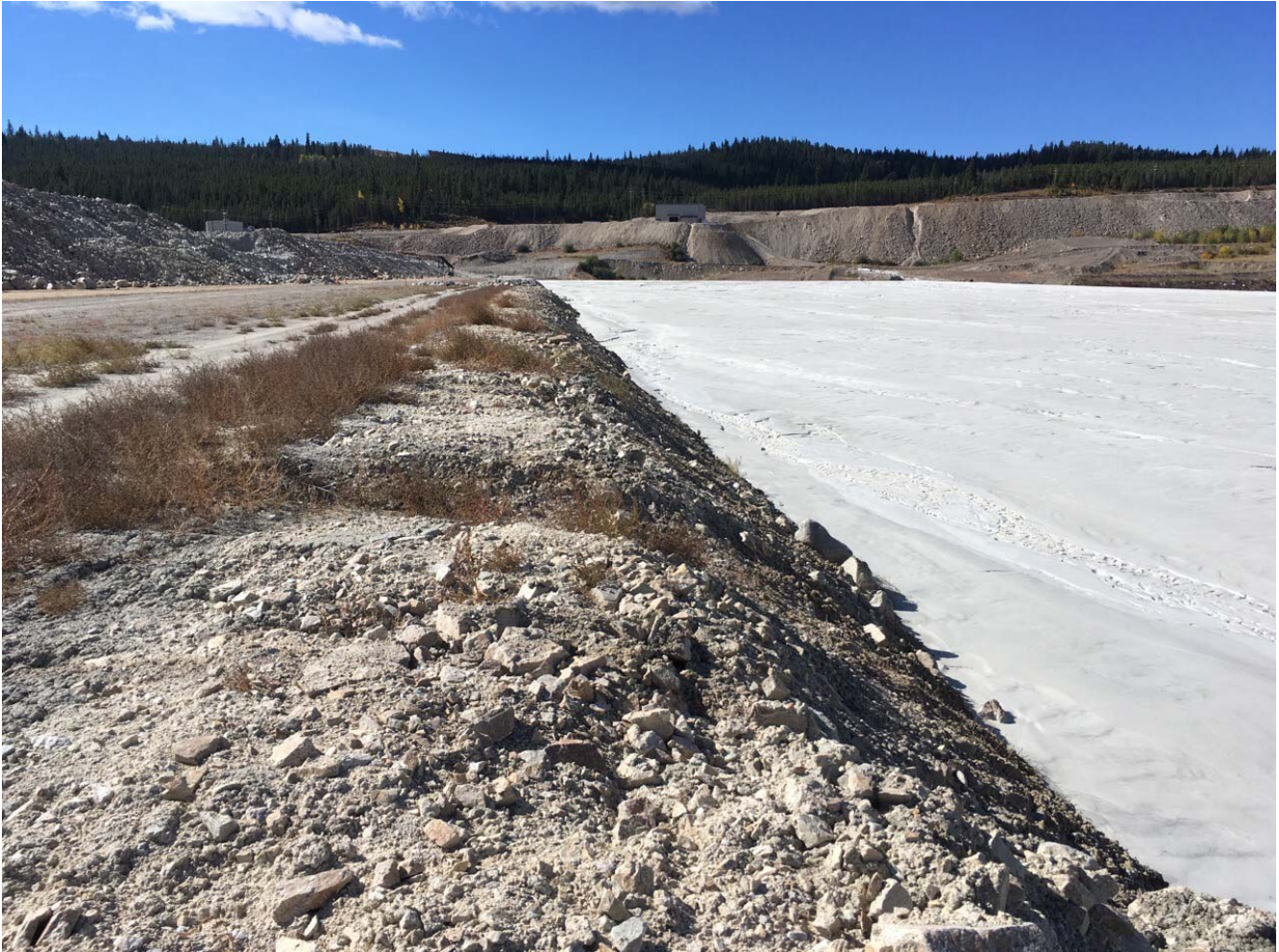
Photo II-B-7 Existing longitudinal crack on downstream edge of SG2 fill zone, with no signs of fresh movement or vertical displacement across crack; crack is >30 cm deep and up to 20 cm wide; hairline crack approx. 1 m upstream of the main crack (HH-2017-07)
