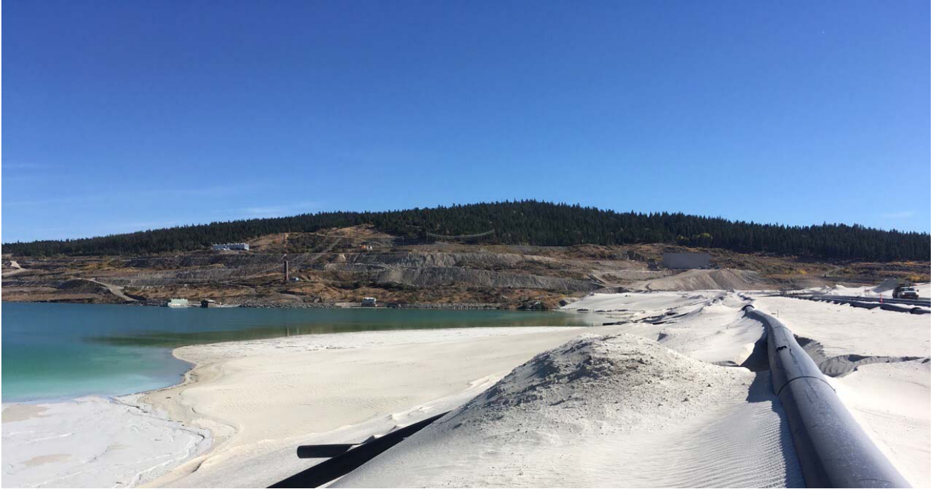
Photo II-A-7 Pond at the Toe of the Upstream Dam Slope – Facing South (LL-2017-09)
