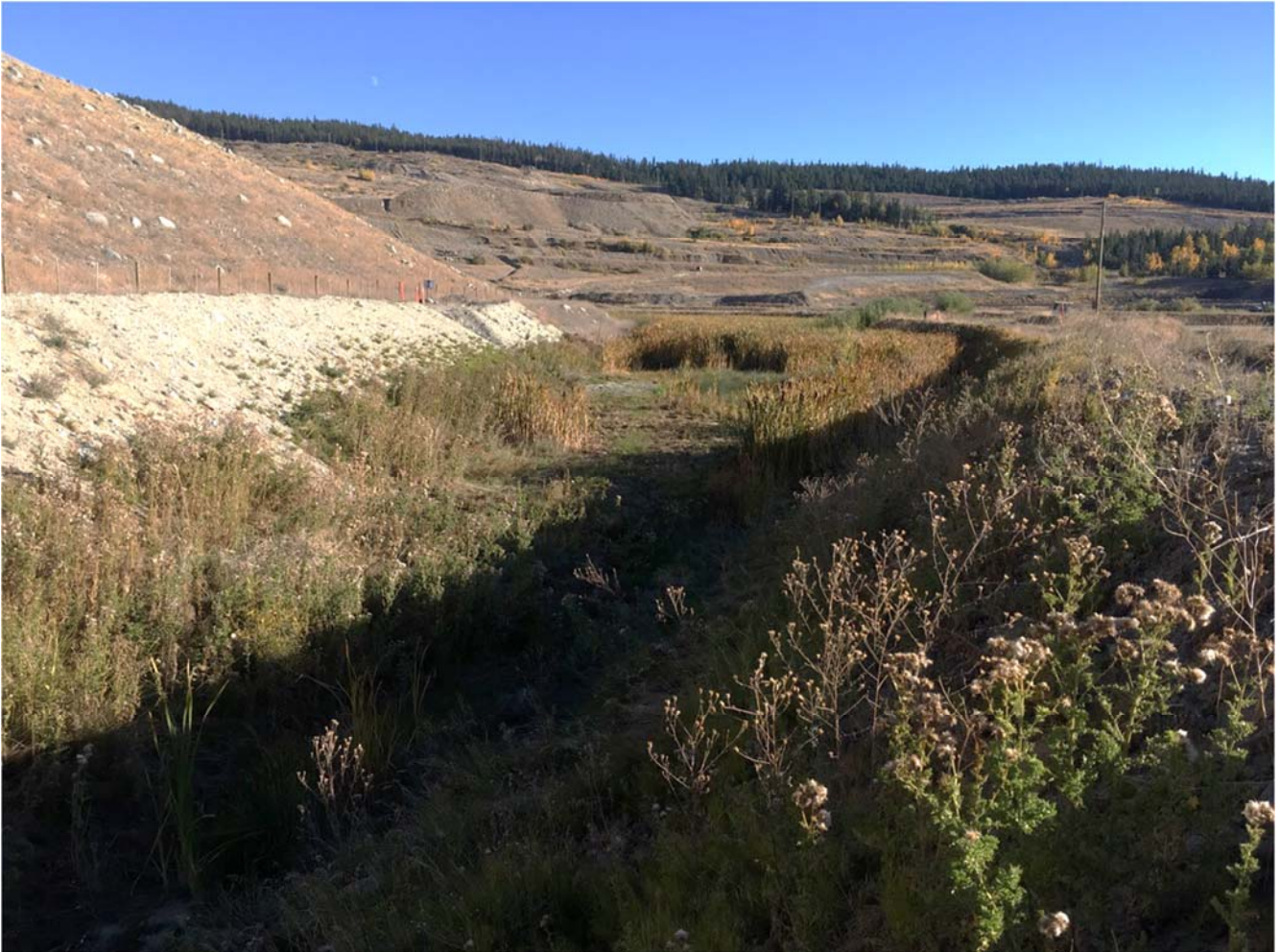
Photo II-A-26 Point A Weir – No Flow, Overgrown by Vegetation and No Longer Functional (KCB3) (LL-2017-23)
