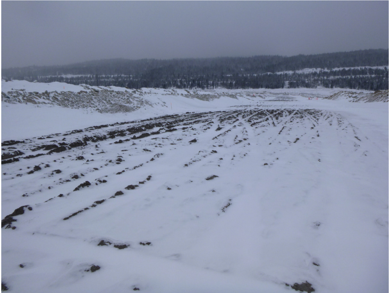
Photo 5 – Sections of the till core zone were heavily rutted (looking northeast).
