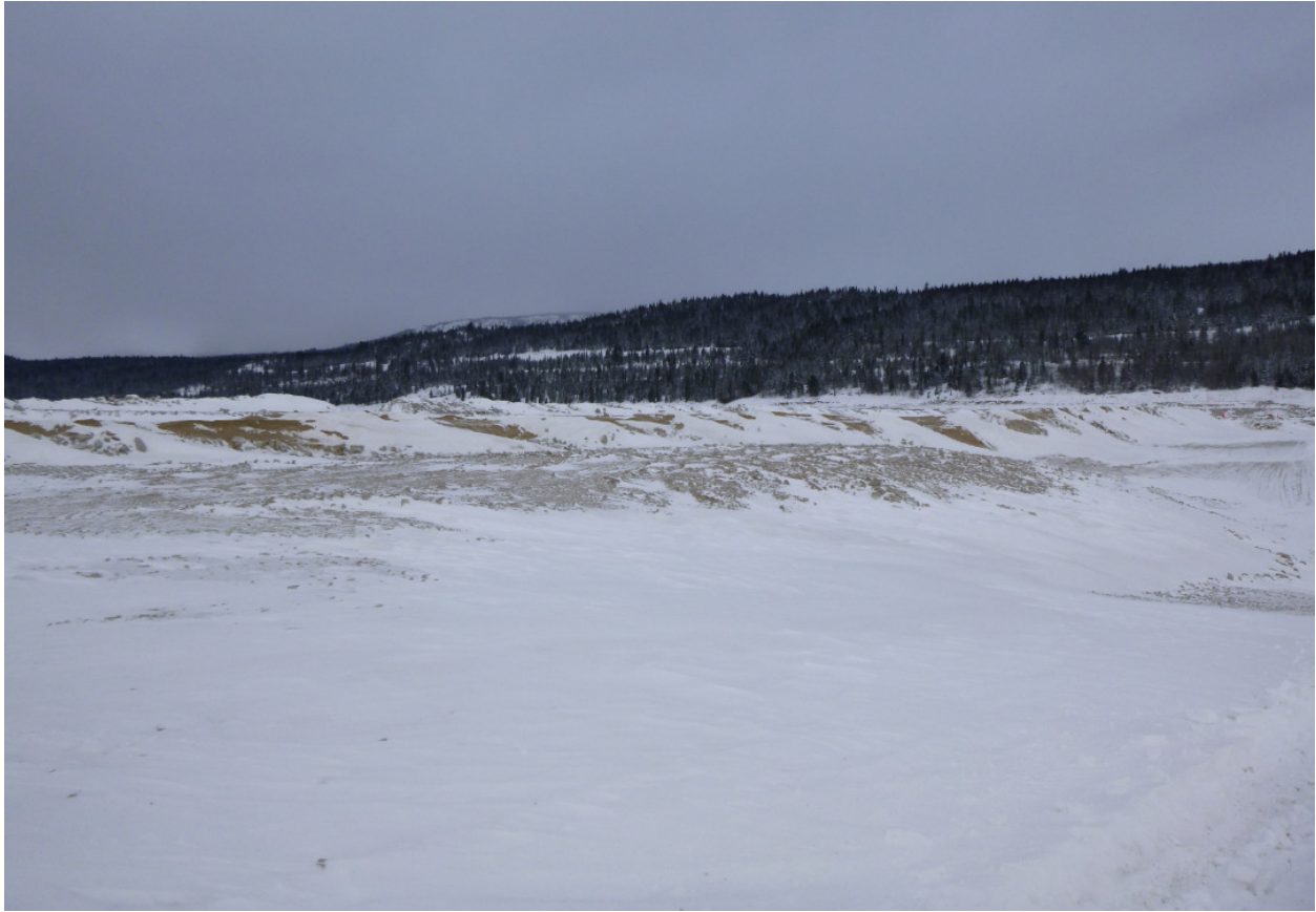
Photo 6 – Area where THVCP Mine Ops hauled, dumped and wheel packed d/s RF2 material from December 8 to 10, 2017. The material was placed between ~Sta. 1+475 to ~Sta. 1+625 to ~El. 1268 m to support and buttress the SG2 where cracking had previously occurred (refer to MRM-2017-004) (looking north).
