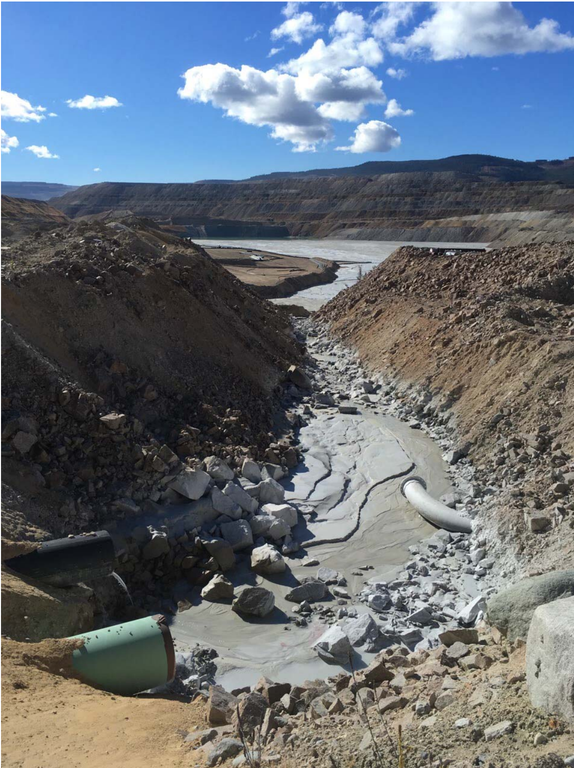
Photo II-D-7 H-H Pumphouse emergency dump outflow pipes, facing southwest (ML-2017-06)
