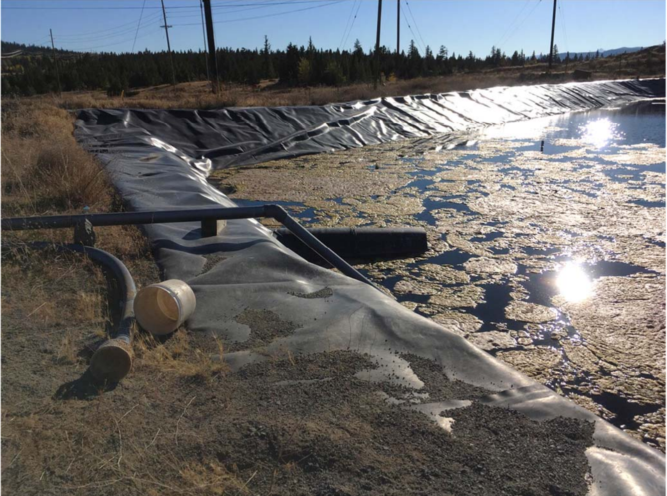
Photo II-C-10 Seepage Pond 2 Outflow Pipe – Facing West; Outlet not yet repaired (SS-2017-08)
