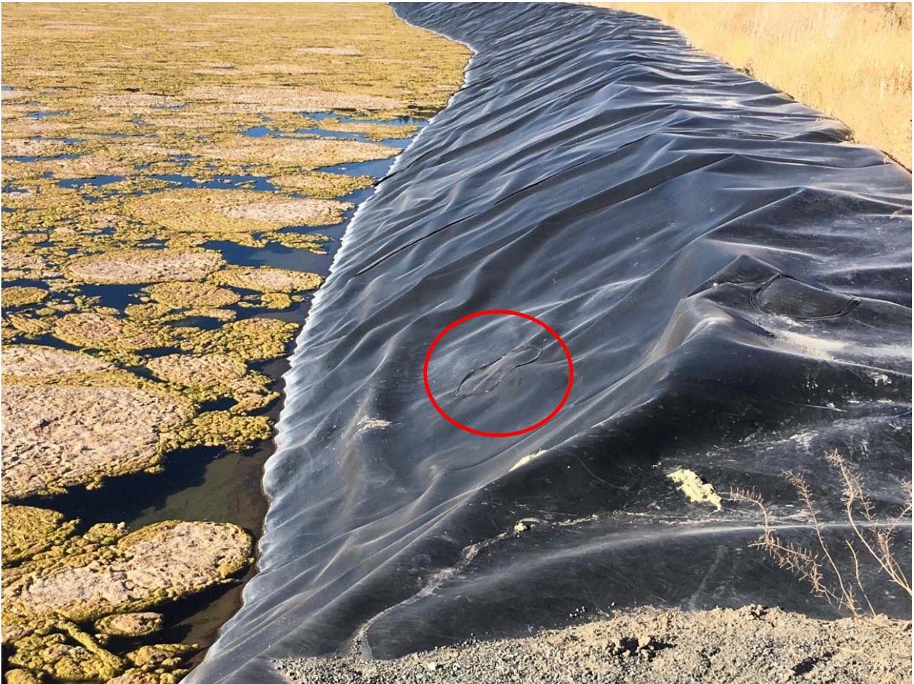
Photo II-C-11 Seepage Pond 2 Tear in Liner Repaired in 2017 – On east side of pond (SS-2017-08)
