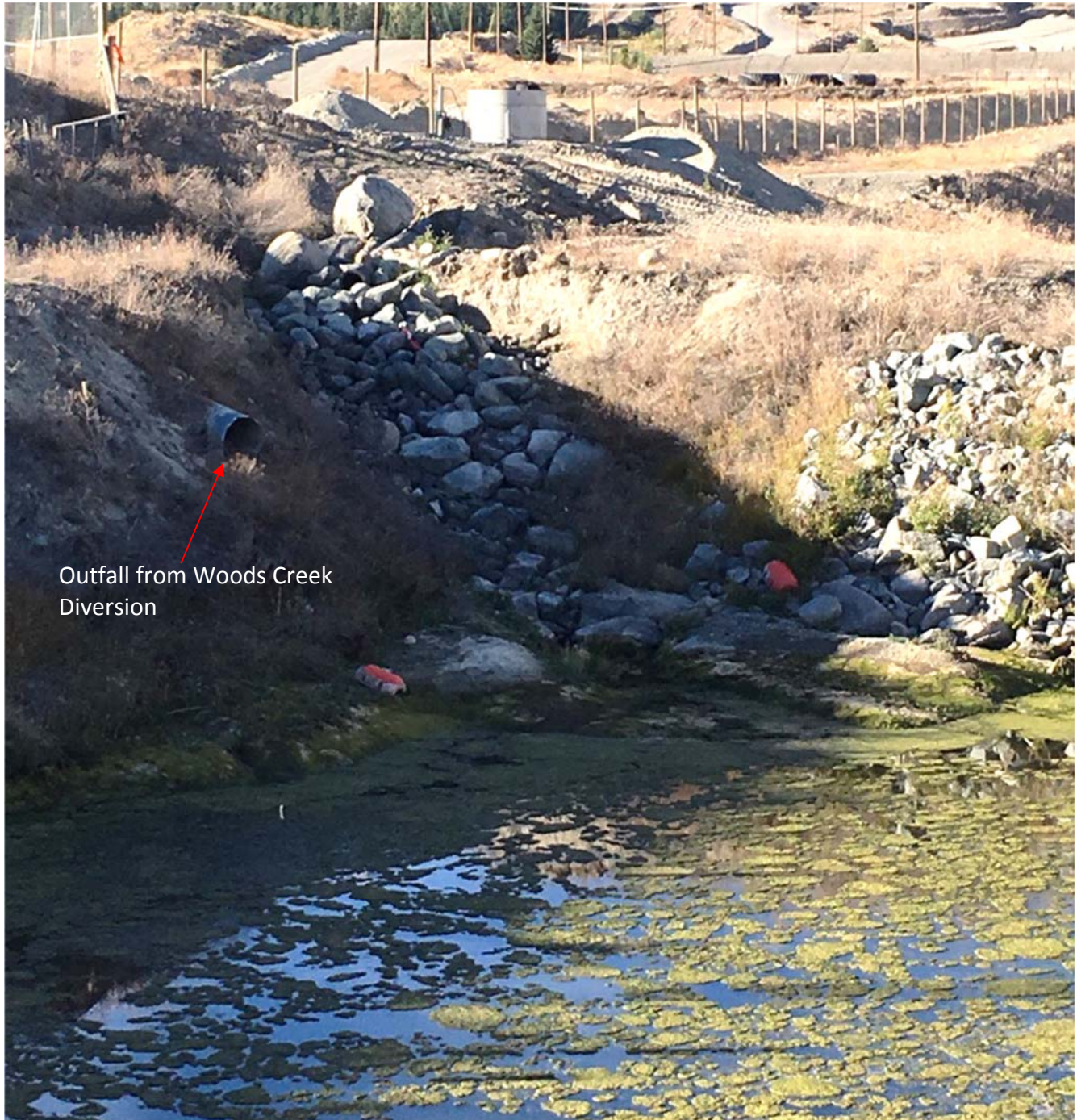
Photo II-C-14 Seepage Water Reclaim Pond – Outfall from Woods Creek Diversion – Facing Northwest (SS-2017-09)
