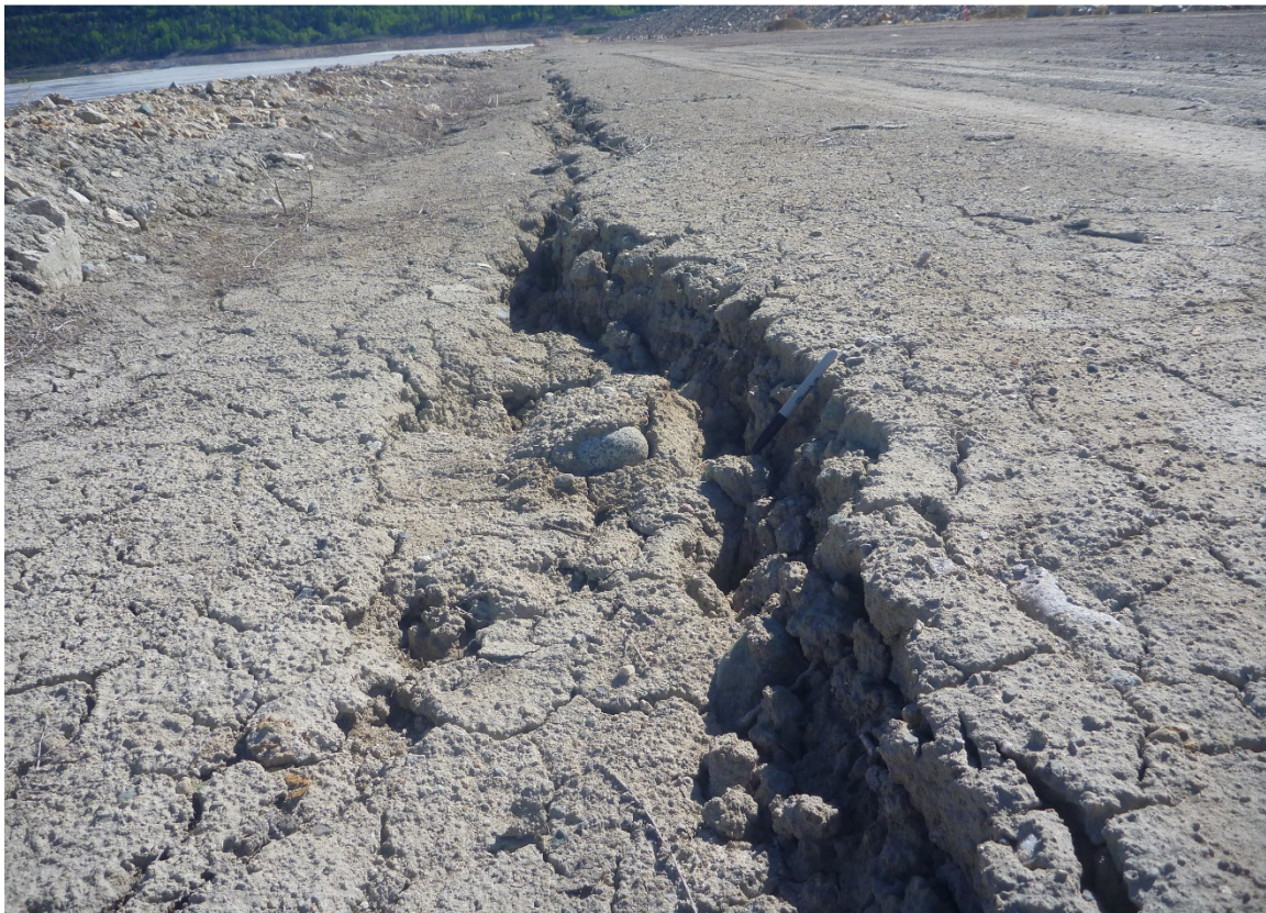
Photo 2 - Cracking at the seam between RF1 and U/S RF2 at approx. Sta. 0+800
